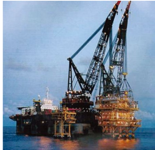
Recovery platforms water supply system
