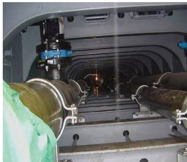
Ningbo ship ballast piping
