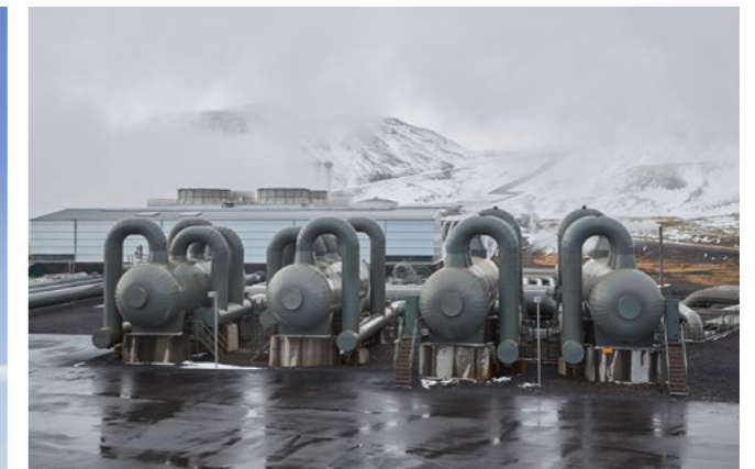
Hot spring pipes
