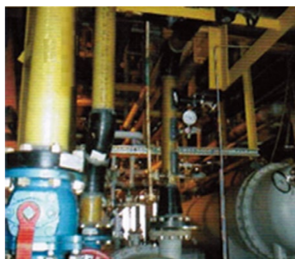
Offshore Oil Field Cooling Water Line for Oil & Gas Pot
