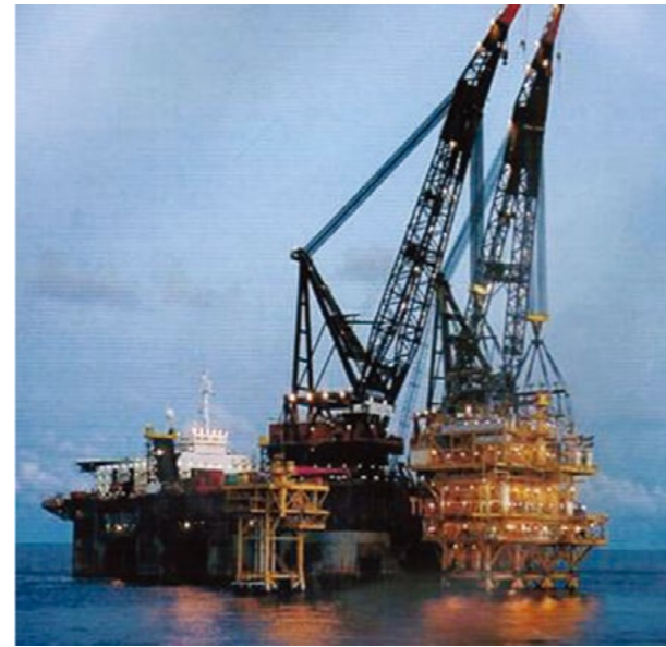
采油平台供水系统 Recovery platforms water supply system
