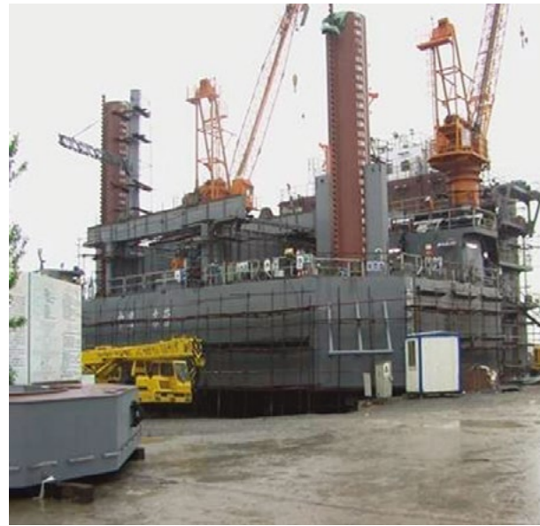
钻井平台酸性气体排放系统 Acid Gas Exhaust System of Drilling Unit Platform
