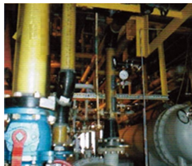
海上采油平台油气储罐冷却水管线 Offshore Oil Field Cooling Water Line for Oil & Gas Pot
